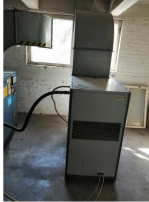
Figure 5: The compressors at the production facility
